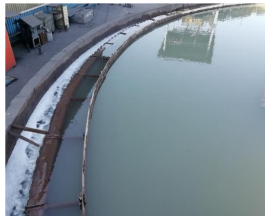
Figure 11. The thickener surface after modification in the operation condition
