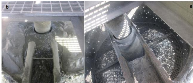
Fig. 4. (a) Pulp and froth overflowing from feedwell (b) blocked openings of the feedwell.
