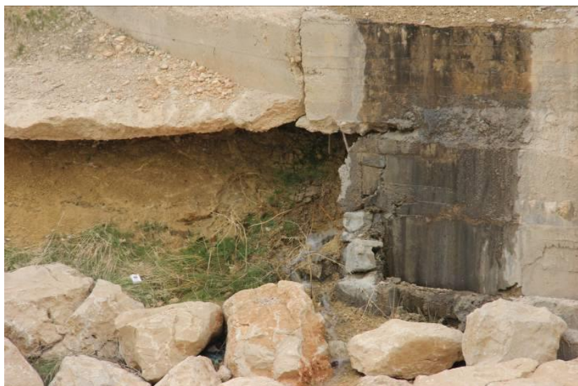
Fig. 1. b) Piping hole and seeping flow between abutment and concrete body at downstream
