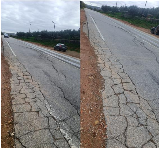
Figure 3. Pavement creep observed at the My Idriss site (N13 road).
