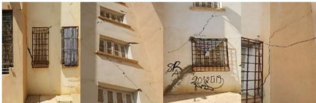
Figure 3. The generated cracks in zone 1.
